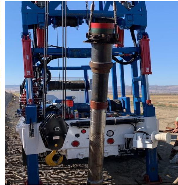
APH Valve Installed Below Pump Bowls
