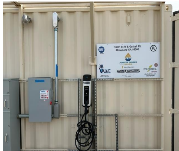
APH Container with EV charger
