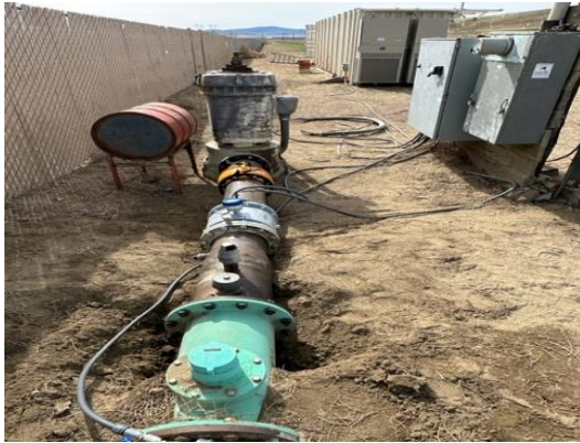
Existing Well Pump to APH
